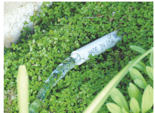
Figure 5 - System Rinse Line
