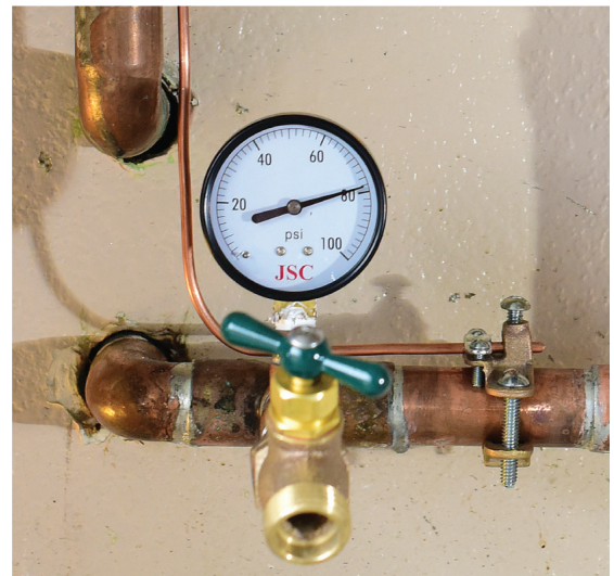
Figure 9 - Copper wire clamped to incoming water main.
