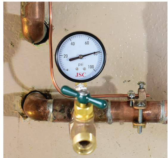
Figure 9 - Copper wire clamped to incoming water main.
