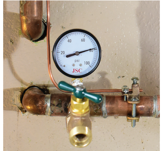
Figure 9 - Copper wire clamped to incoming water main
